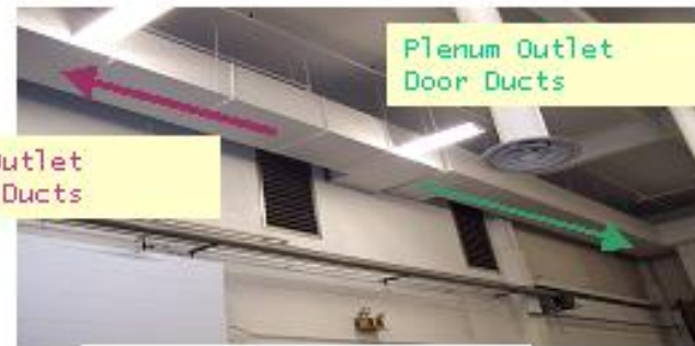
West Terminus of Solar Heating Plenum
