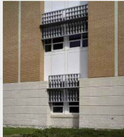
West Facing Solar Shading Screens
