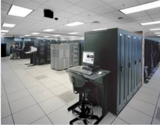
4th Floor University Data Center
