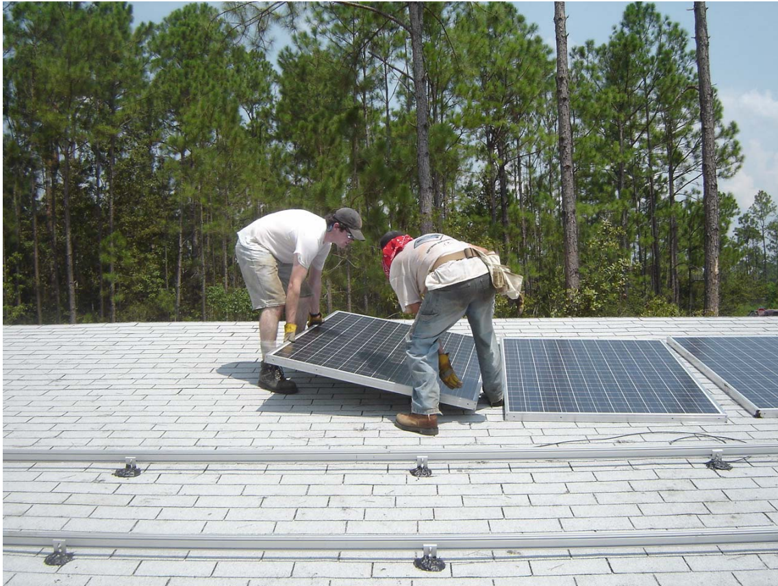
Paxton Marshall's students prepare to install PV panels on ecoMOD house designed and built by UVA students for a family in Mississippi that lost its house to hurricane Katrina.
