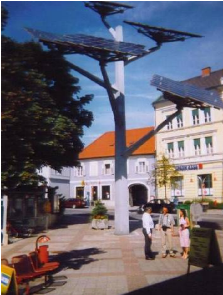
Solar Tree, 22 KW, Geisdorf, Austria
