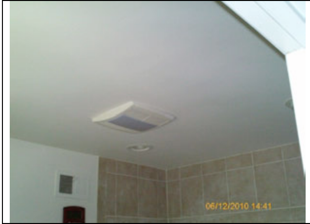
Fan exhaust to attic
