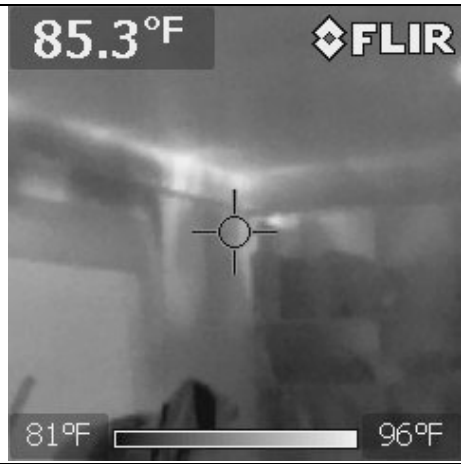
Top plate air sealing needed
