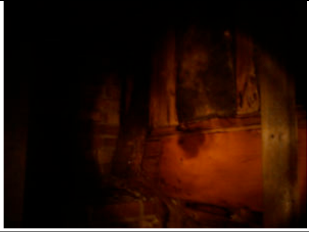
Dirty insulation from air movement
