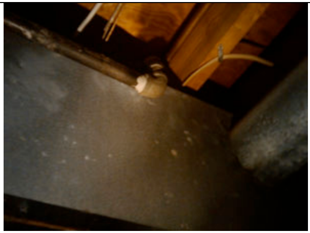
Small gas leak detected – have checked by licensed plumber/gas fitter
