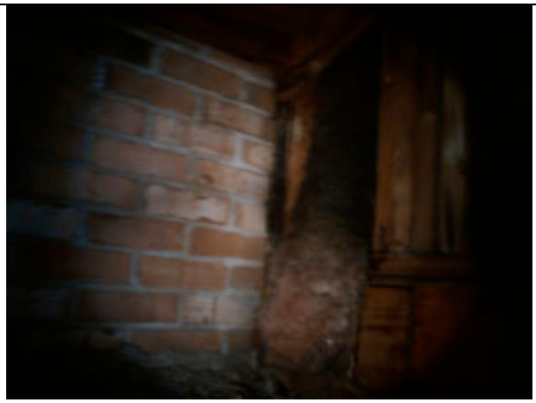
Thermal bypass from living space to garage attic
