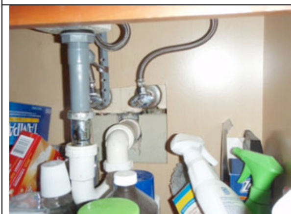
Air leakage at plumbing penetrations
