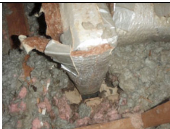
Thermal bypass at duct penetration
