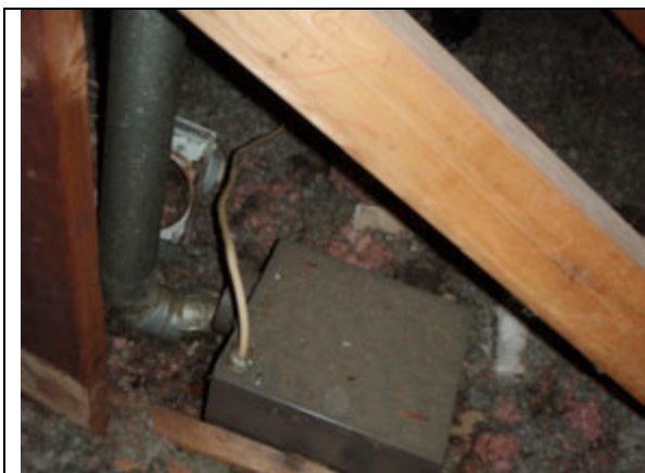
Disconnected bath exhaust fan
